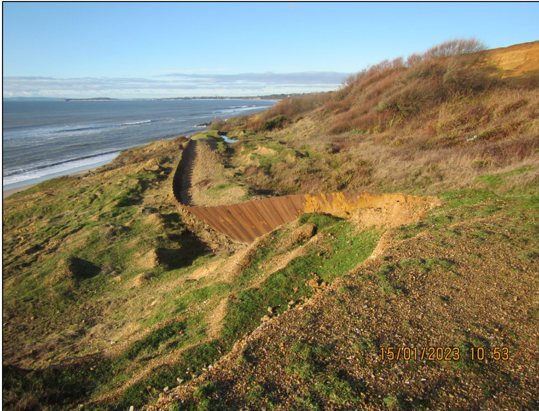
Photo of the lower cliff at Barton on Sea, showing the failed sheet pile wall and drainage system in the active land slide section, opposite Barton Drive (Source: Courtesy of New Forest District Council).
