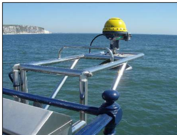
Figure B.14 WaveRadar REX on Swanage Pier
