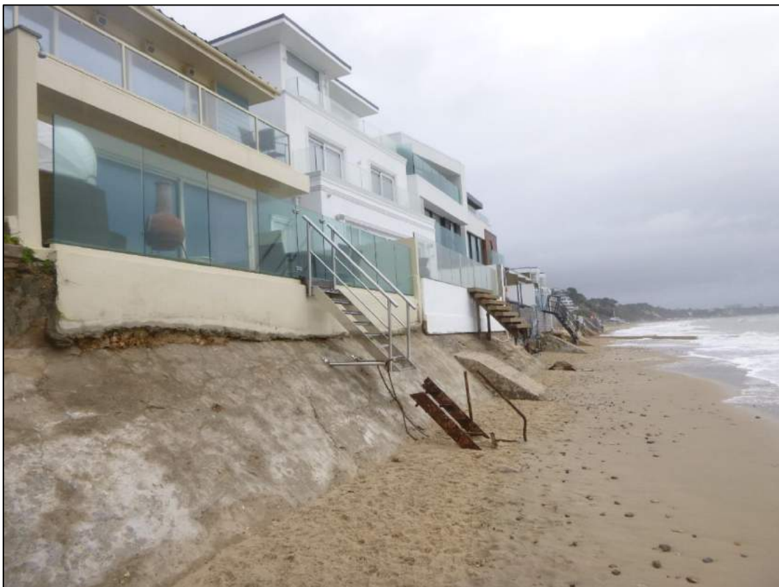
Figure B.1 Beach erosion at Sandbanks following the winter 2013 to 2014 storms left the beach denuded of sand
